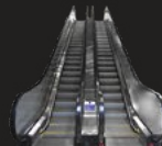
Escalators and moving walkways
