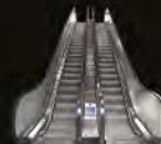
Escalators and moving walkways
