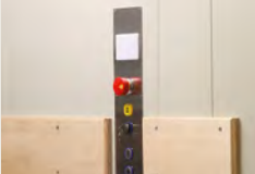
Lift car operating panel
