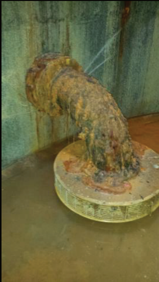
Pump suction outlet pipe work and anti-vortex device, showing signs of heavy corrosion to the pipe elbow.
