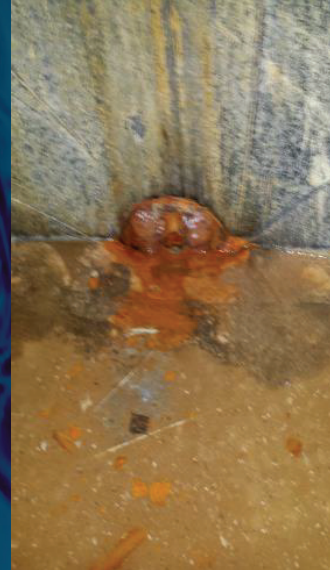
Drain valve. Severe corrosion
