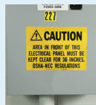
Hazard warning signs
