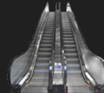
Escalators and moving walkways
