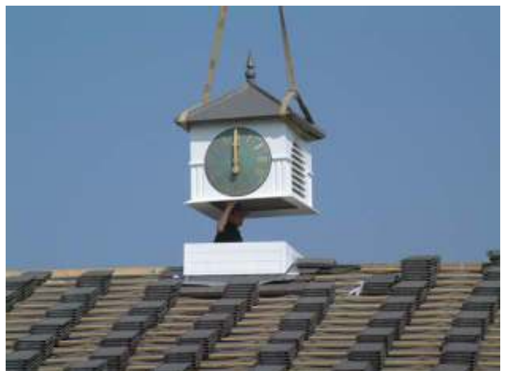
Cupola being lowered in to position. The use of a crane is recommended on cupolas over 900mm wide.
