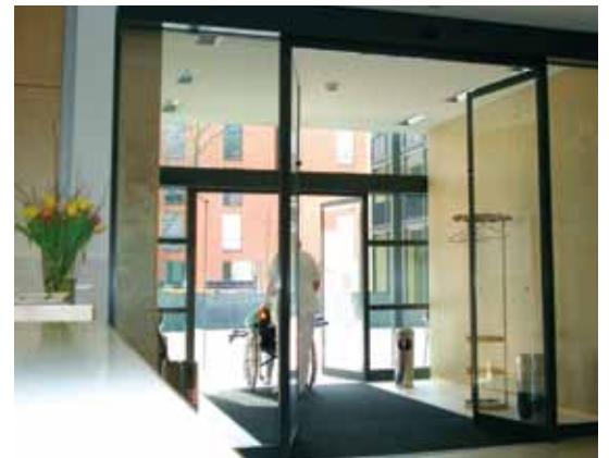
Automatic redundant sliding door with emergency opening system
