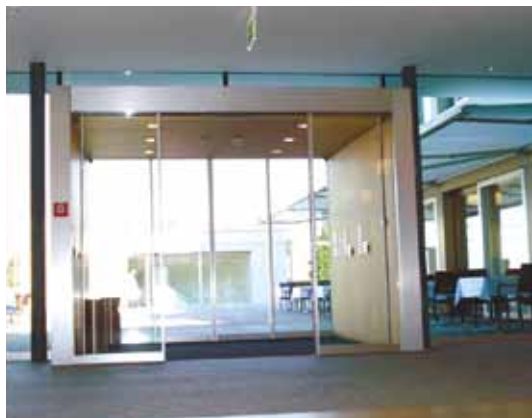
Double automatic sliding doors, draught lobby
