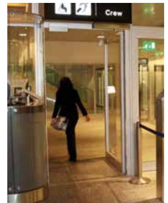
Revolving door operator, crew entrance, ZRH
