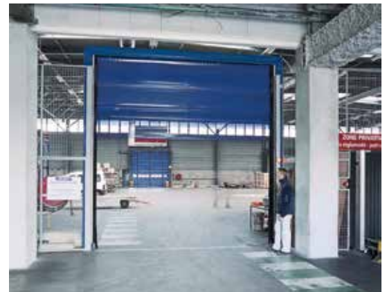
Automatic rapid shutter door, hangar, LYS
