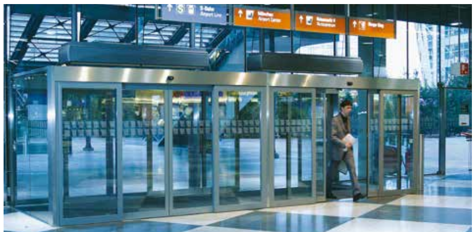
Smoke-protection doors, entrance area, MUC
