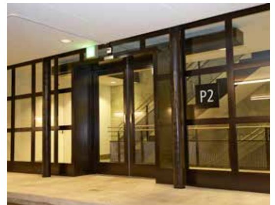
Automatic fire-protection door, multi-storey car park
