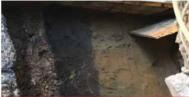
HYDROCARBON LAYER FOUND AT RESIDENTIAL PROPERTY
