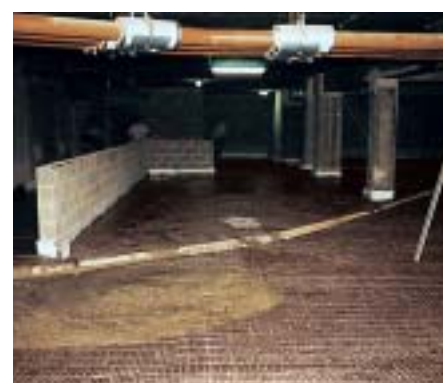
European Building, Brussels: The entire underground garage was put at risk by fluctuations in the groundwater level.
