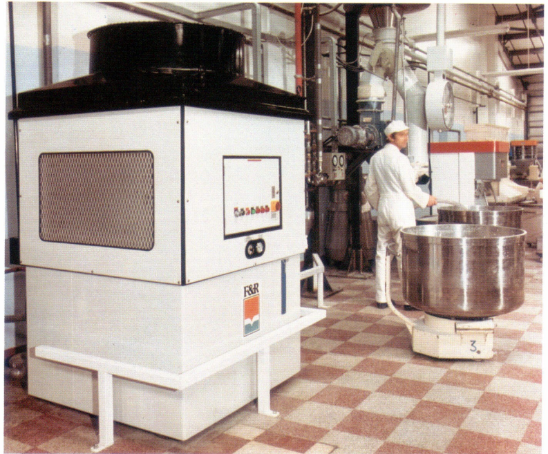
RCU 8-PB supplying chilled water at 1°C to control dough temperature at mixing stage.
