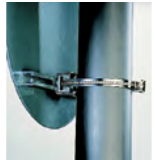
Rear of traffic sign showing stiffening channelling.
