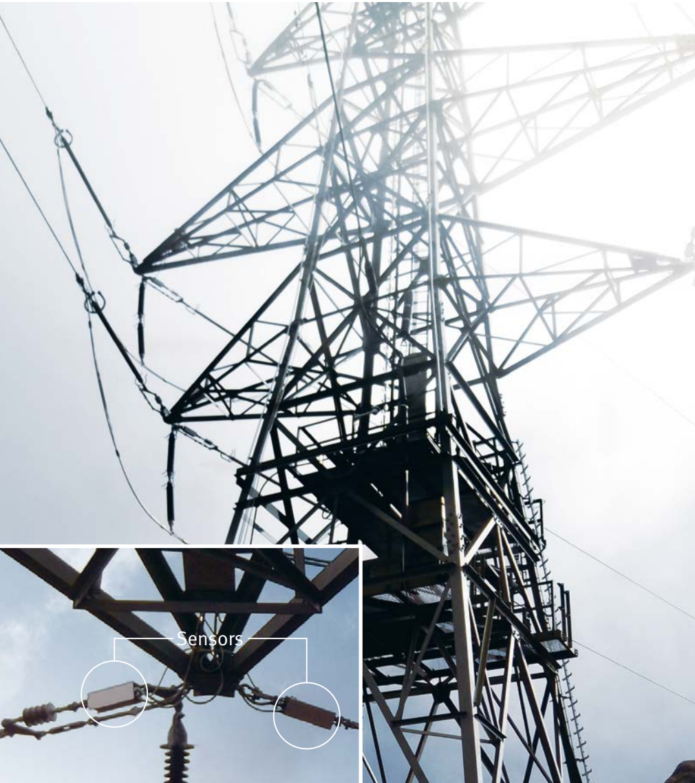
The ice load is measured at especially critical points by strain gauge sensors attached to the masts
