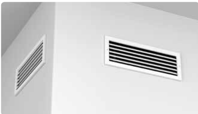
Fig. 3: The Approved Code of Practice (ACOP) L8 offers guidelines for the prevention and treatment of legionella in HVAC systems.
