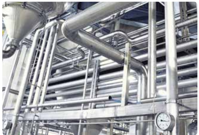
Fig. 4: Hot-water pipes up to 70 °C in temperature can help to eliminate legionella.
