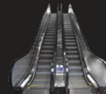
Escalators and moving walkways
