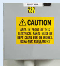
Hazard warning signs
