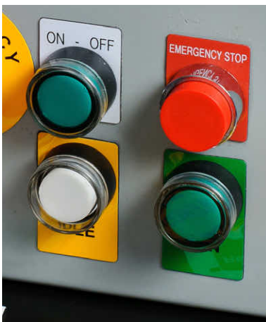
Control panel labels
