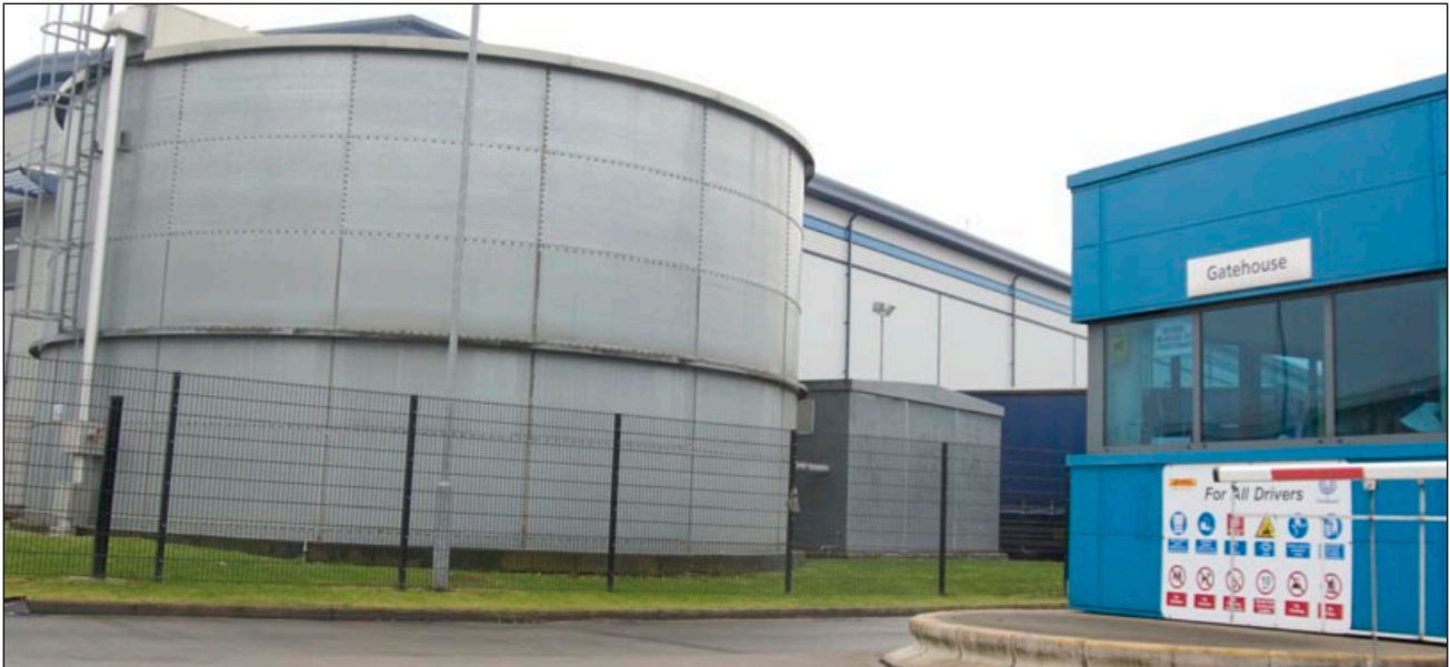
Figure 42 A firewater tank
