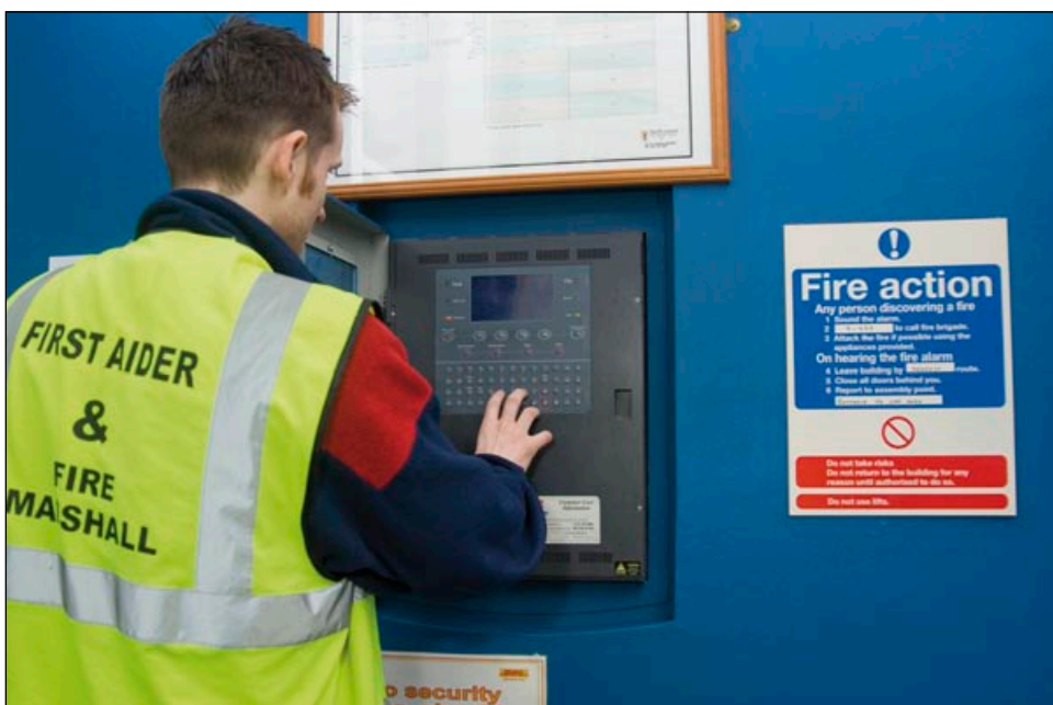
Figure 38 A fire marshal monitoring the fire alarm system
