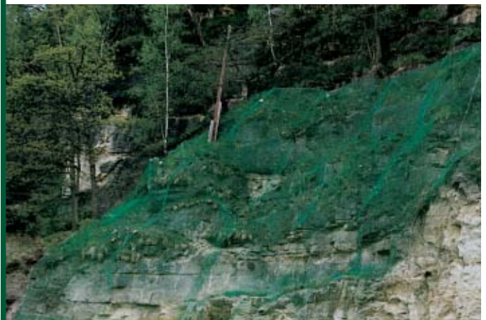
No. 209-045-01 Embankment safety nets
