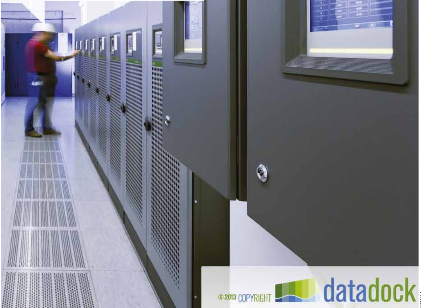
Datadock data centre: 8 x 200 kVA DELPHYS GP UPS.
