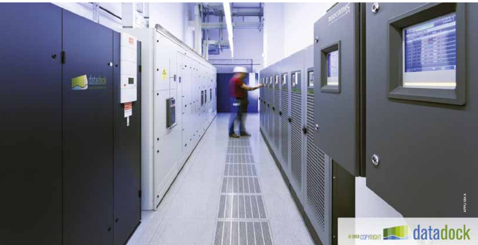
Datadock data center: 8x200 kVA Green Power 2.0 DELPHYS GP UPS and BHC battery monitoring system.
