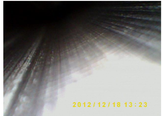
Endoscopic Image showing internal pipe after pigging
