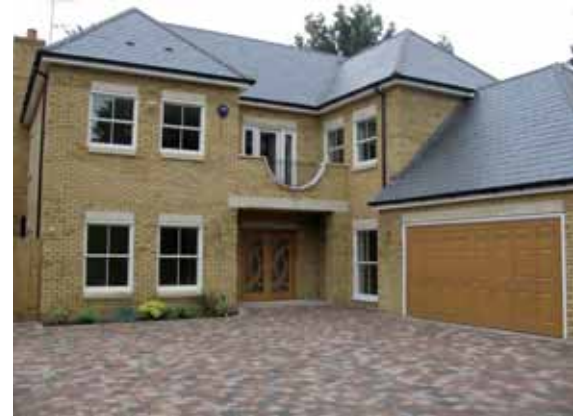
Standard H1 Window Heads with C3 Slip Cills, C220 Once Weathered Coping including Vertical Curve and Special Structural Front Door Lintol. (DCM)
